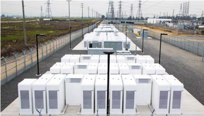
Tesla's 129 MWh installation ($50M)
